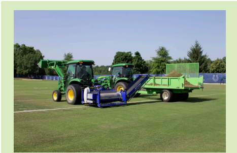
Fraze mowing involves a special tilling machine that removes the top layer of the turf and leaves the roots, rhizomes, and some crowns, depending on the height of the mow.
