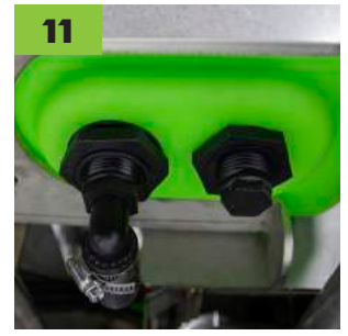
Tank Sump with Drain
